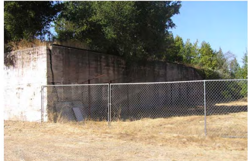
Main House/Faculty Residence ruin, retaining wall that supported a west portion of the house.
