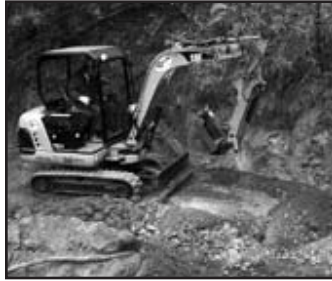
Mark Casaretto on an Excavator Finishing Work on a Culvert Installation Project
