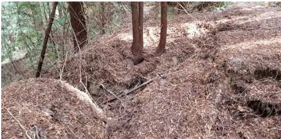
Photo 4: Partially washed out fill crossing
