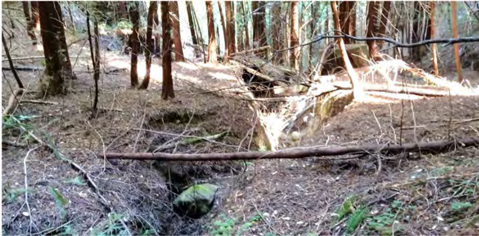
Photo 13: looking downstream at the partially washed out Humboldt crossing. Stream flow drains underneath a fallen stump just to the left of the eroded channel.
