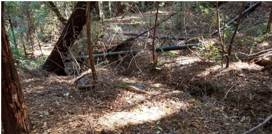
Photo 3: Partial washed out fill crossing
