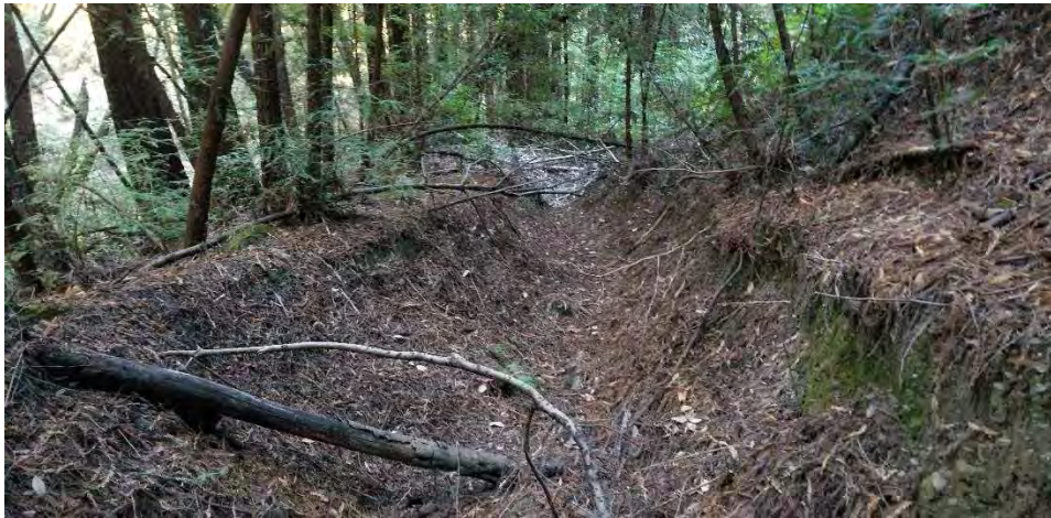
Photo 14: looking down the road at the eroded channel from diverted stream flow. This photo was taken along the lower portion of the gully where the incision is much greater. Note the heavy duff layer in the channel bottom.
