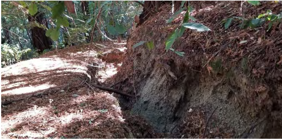
Photo 2: Gully from diverted watercourse down skid trail
