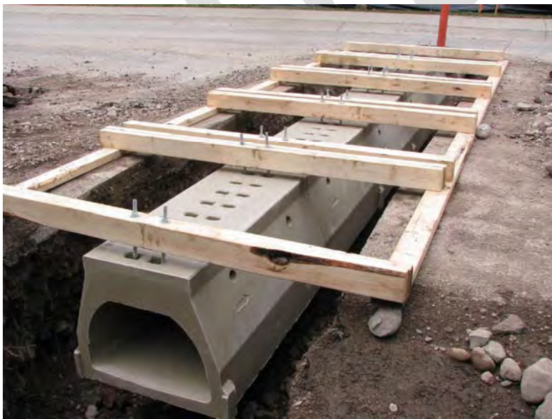
Herp (amphibian and reptile) crossing under construction - Waterton National Park, Alberta, Canada
