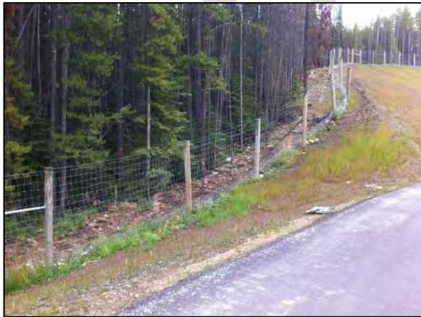
Example of directional/exclusion fencing – wire at top is to help deflect falling branches
