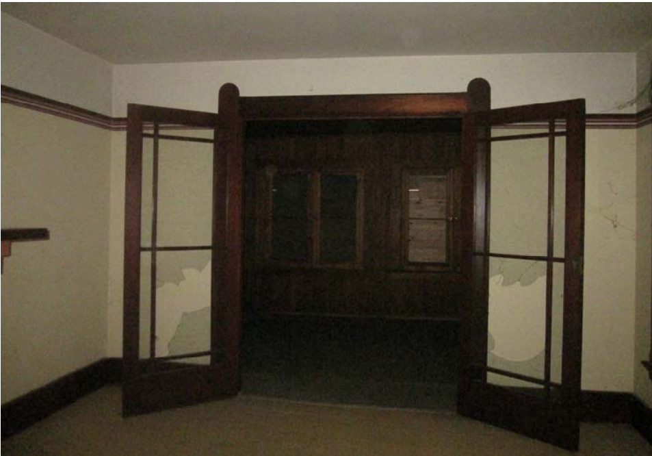
Below: Typical woodwork and the French doors at the upstairs Master bedroom. Photograph B. Maley, March 2013.
