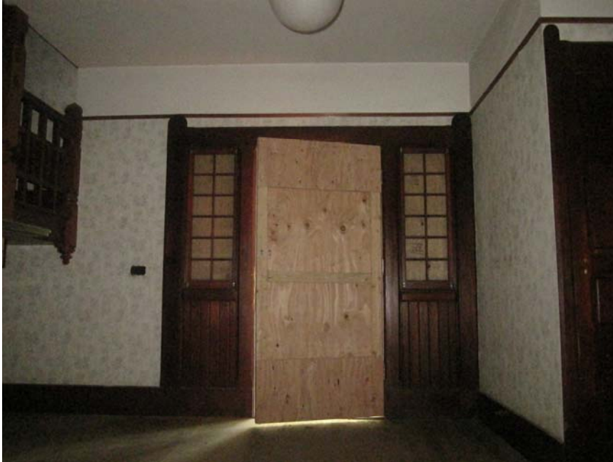
An interior view of the main doorway with sidelights. Photograph B. Maley, March 2013.
