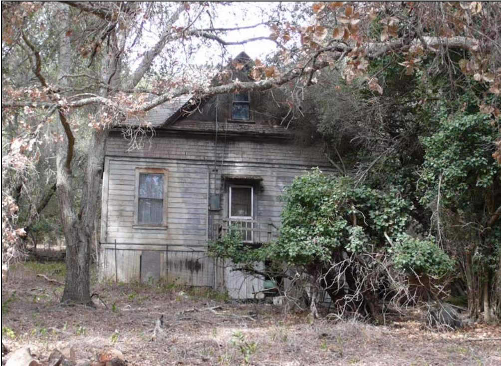
The simple, center gabled dormer set within a hipped roof gives the Cottage the feel of a small, Carpenter Gothic cottage. Image from Portola Valley Town Archive, August 2008.
