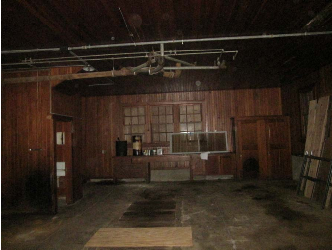
The downstairs of the garage showing the wall of built in cabinets. Photograph B. Maley, March 2013.
