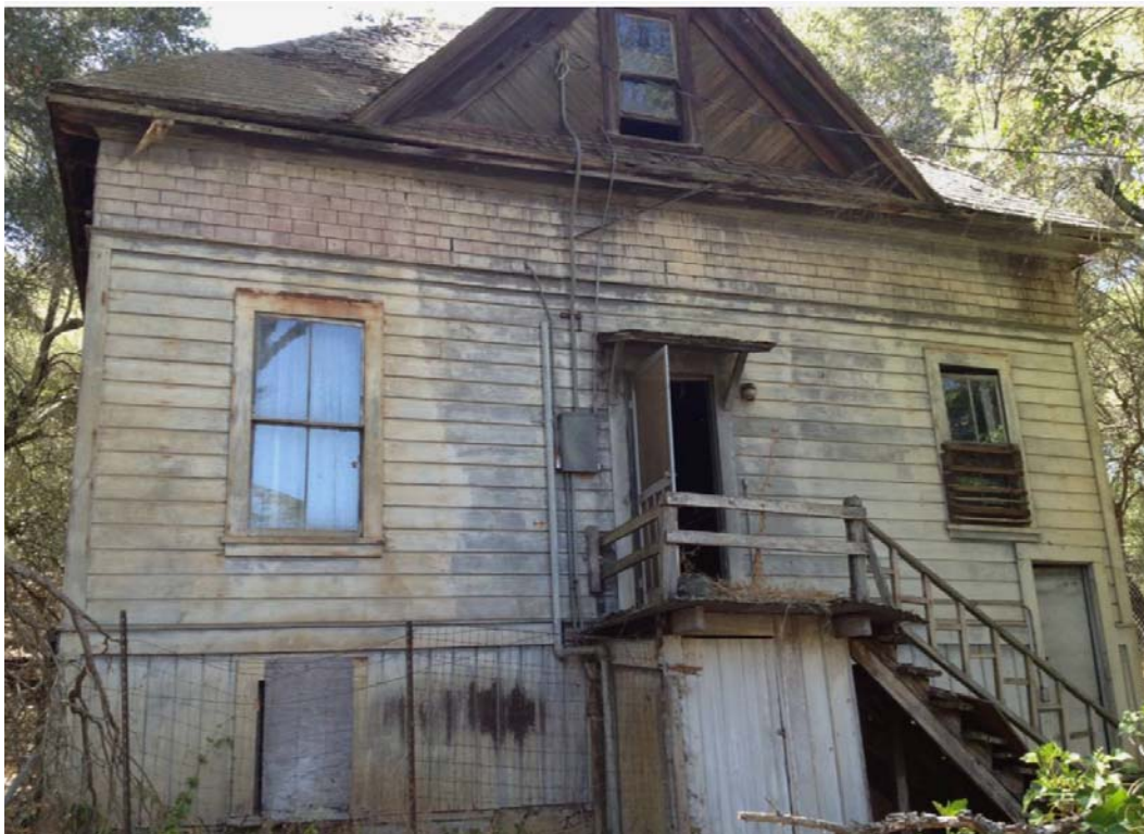
The front (east) elevation of the Cottage in 2012 (before boarding of windows and doors) showing its steeply pitched dormers, exterior siding, windows, and front stair.
