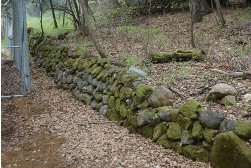
The retaining walls (stacked field stone) along the upper and lower sides of the terrace northwest of Hawthorn House. Photograph Denise Bradley, March 2013.
