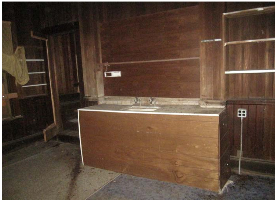
The interior of the Cottage, showing the alterations that have occurred. Photograph B. Maley, March 2013.
