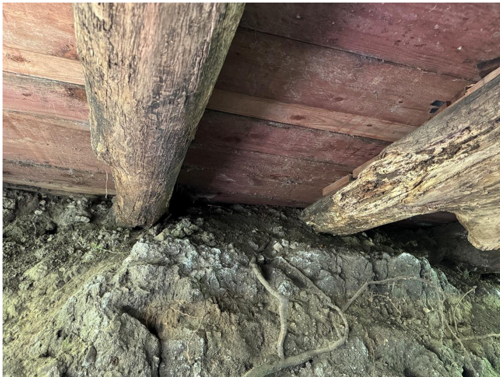
Figure 7. Detail: Log stringers deteriorating.
