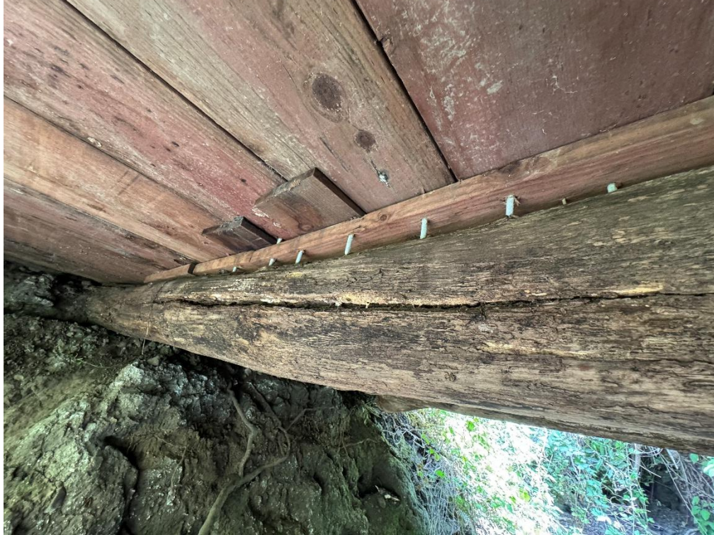
Figure 6. Detail: deck separating from girder.
