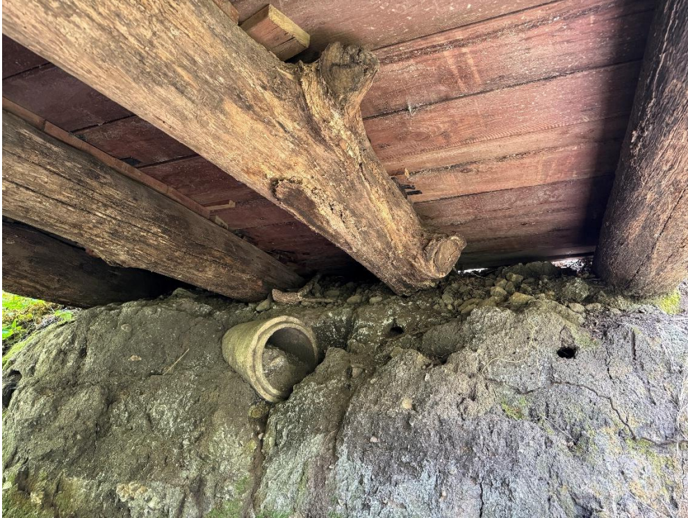
Figure 4. Log supported deck; non-existent footing, eastern end.
