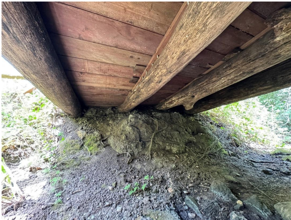
Figure 5. Log girders and stringers; non-existent footing, western end.
