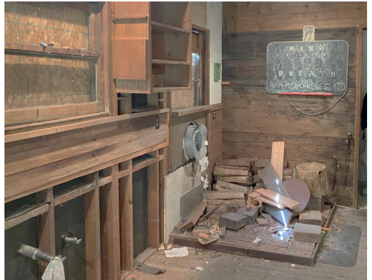
Interior (missing cabinetry and counters)
