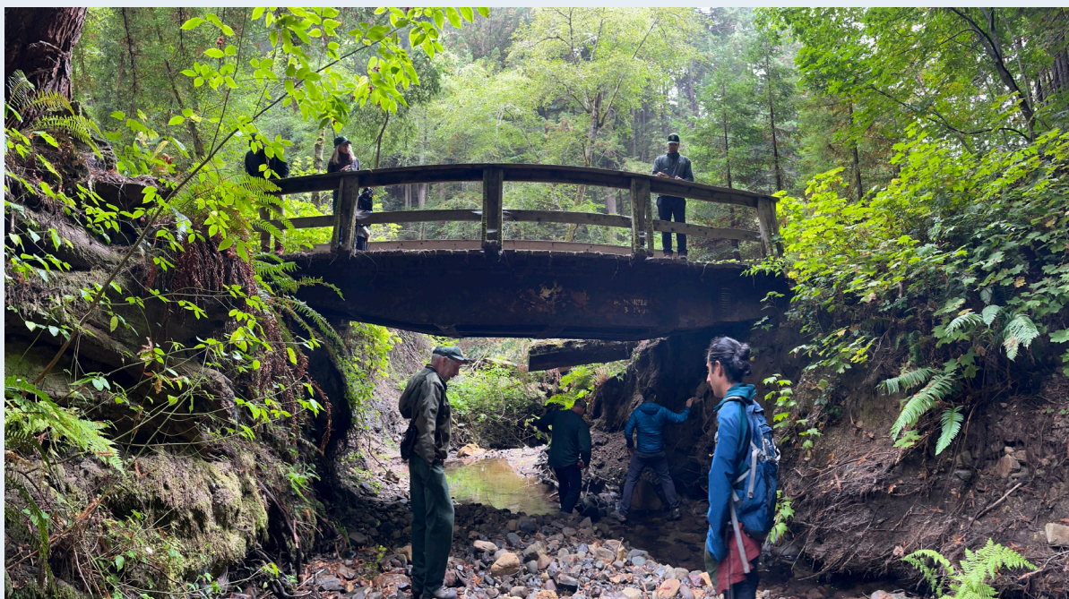
FEMA and Midpen staff inspect washout damage along Purisima Creek Trail, where repairs are needed to restore patrol and emergency vehicle access following the 2022–23 winter storms. Purisima Creek Redwoods Open Space Preserve (Midpen Staff)
