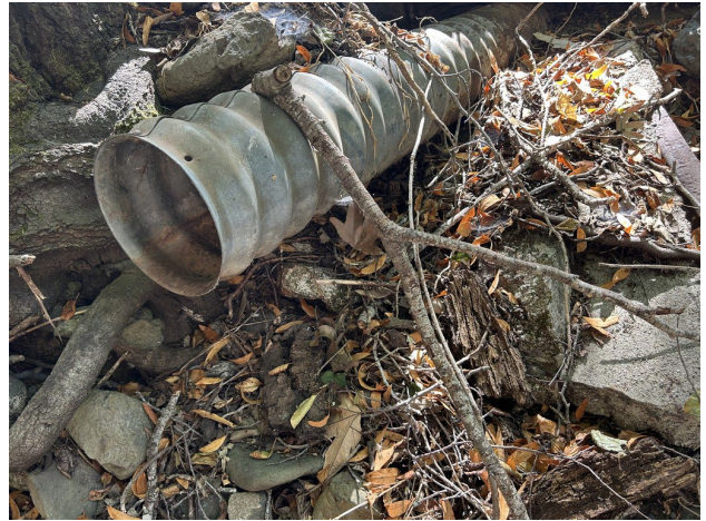
H6: Abandoned corrugated metal pipe.
