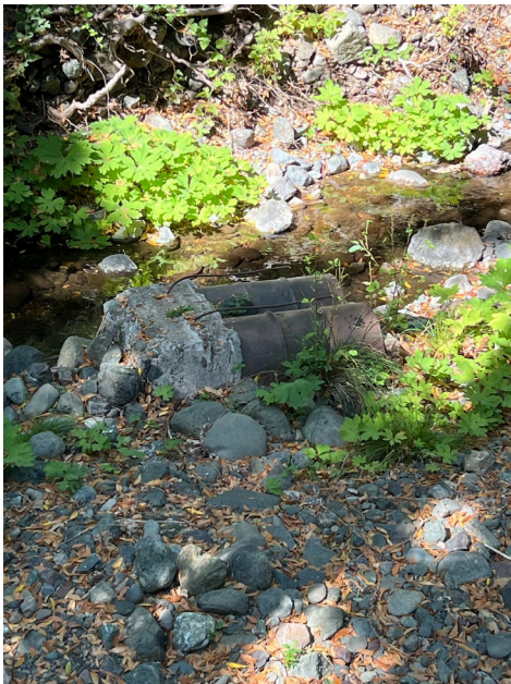
B12: Abandoned corrugated pipes in creek corridor.
