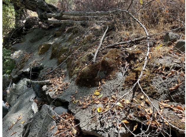
H19: Deteriorated shotcrete and concrete debris.
